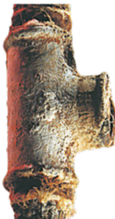
External corrosion - Steel
